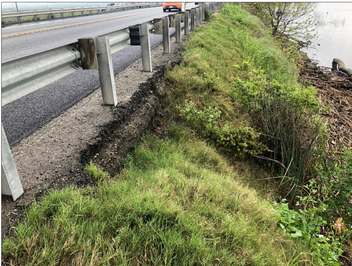
Figure 13. Highway 160 Erosion, Sta. 948+50
