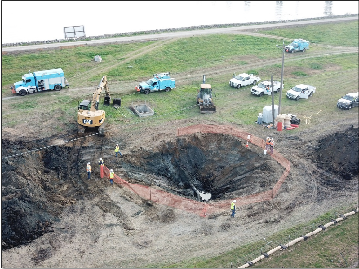
Figure 14. Exposed Fractured Natural Gas Line, Sta. 478+00
